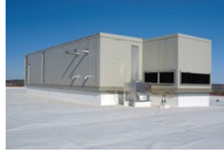
Packaged Rooftop Units
