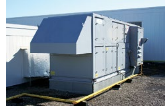
Energy Recovery Units
